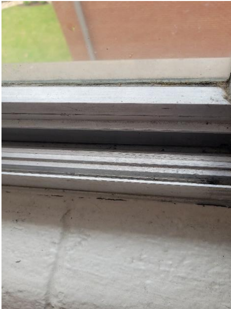
Photo #17 Asbestos-Containing Interior Window Glazing (Dorm Floors) (HA 40)
