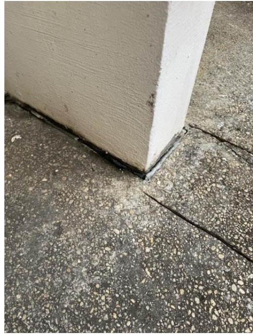
Photo #34 Asbestos-Containing White Wall Caulk (Bottom of Wall) (E15)
