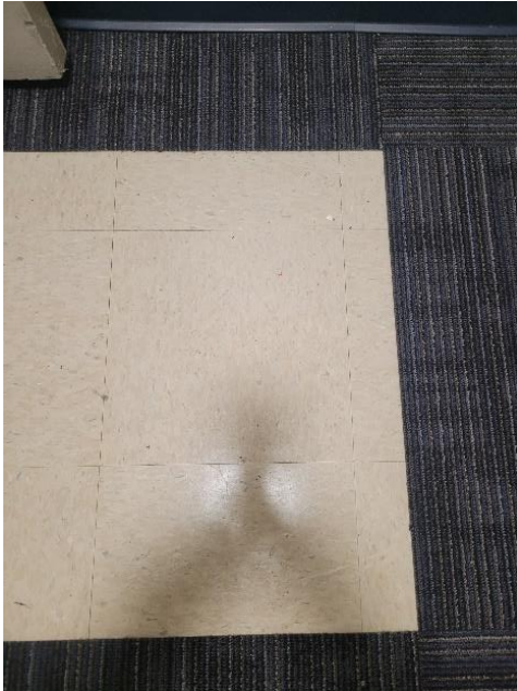
Photo #9 12"x12" White Floor Tile and Mastic and Asbestos-Containing Flooring Below (Under Carpet) (HA 27)
