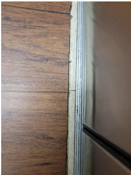
Photo #19 12"x12" Beige Floor Tile with Brown Streaks and Asbestos-Containing Black Mastic under Wood-Grain Plank Flooring (HA 51)
