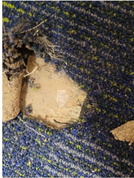
Photo #14 <1% Asbestos Carpet Glue associated with Rolled Carpet (Dorm Floors) (HA 34)
