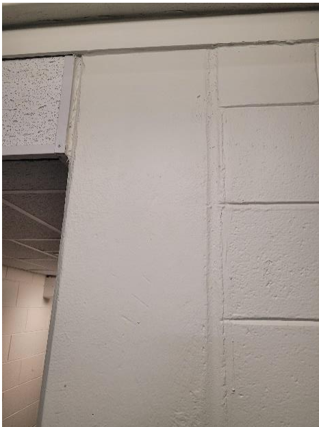
Photo #3 Asbestos-Containing Texture Material (Concrete Walls/Columns) (HA 4)
