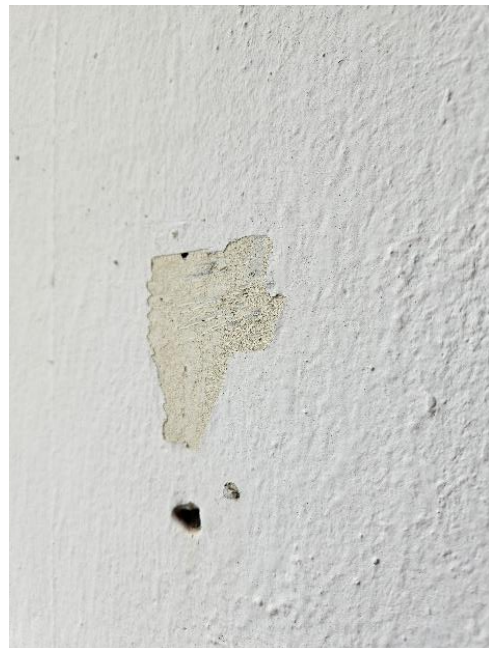
Photo #28 Asbestos-Containing Tan Skim Coat (Under HA E1) (HA E2)
