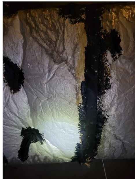
Photo #20 Asbestos-Containing Black Mastic on HVAC Ductwork (HA 56)
