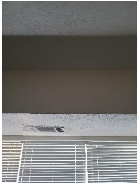
Photo #2 Asbestos-Containing Soffit Surfacing (HA 3)
