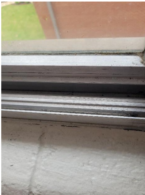
Photo #15 Asbestos-Containing Interior Window Caulk (Dorm Floors) (HA 38)
