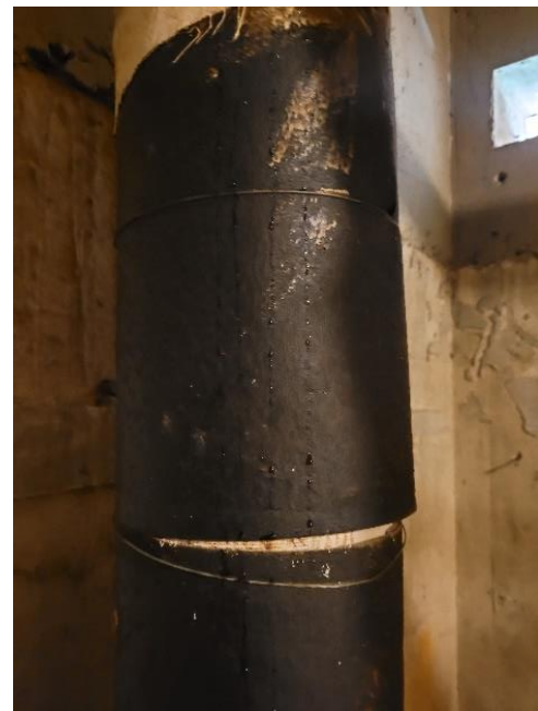
Photo #24 Asbestos-Containing 8" Pipe Black Felt Paper/Tar and Insulation (HA 74)
