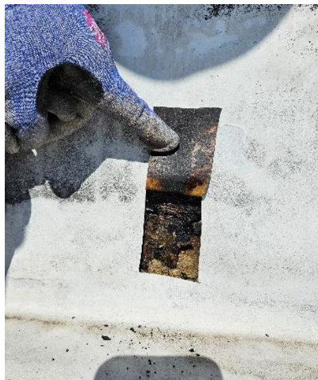
Photo #36 Asbestos-Containing Roof Flashing (HA R8)
