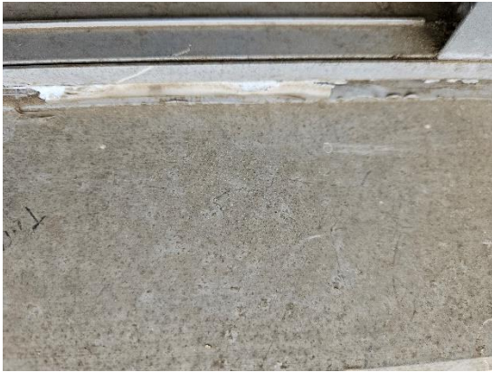
Photo #29 Asbestos-Containing White/Grey Exterior Window Caulk (HA E3)
