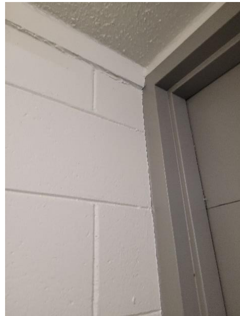
Photo #4 Asbestos-Containing CMU Block Surface Filler (HA 5)
