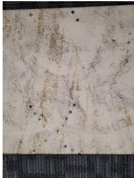
Photo #12 Asbestos-Containing Black Mastic and Leveling Compound on Concrete Under Carpet (HA 31)
