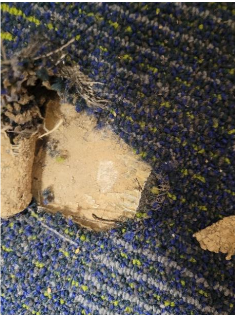
Photo #7 Asbestos-Containing 9"x9" Off-White Floor Tile with White Streaks and Black Mastic (Under Carpet) (HA 25)
