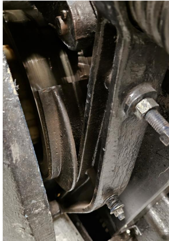
Photo #38 Assumed Asbestos-Containing Elevator Pulley Brake Pad
