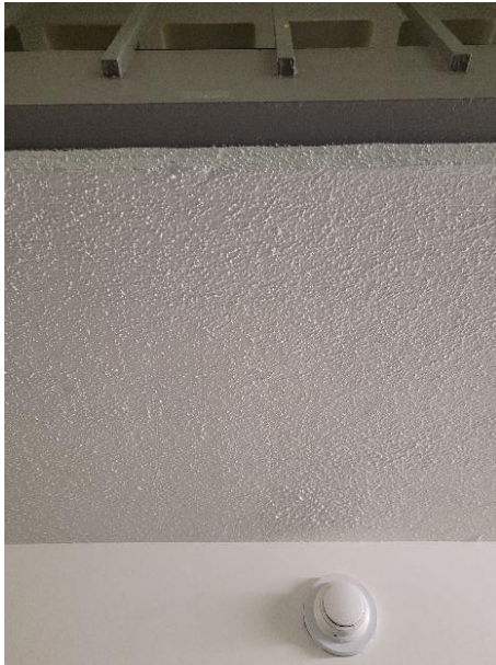
Photo #1 Asbestos-Containing Texture Material (Ceilings) (HA 1)
