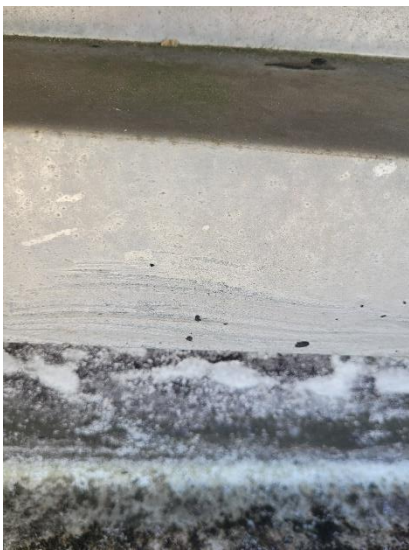
Photo #35 Asbestos-Containing Silver Coating (Roof) (HA R5)
