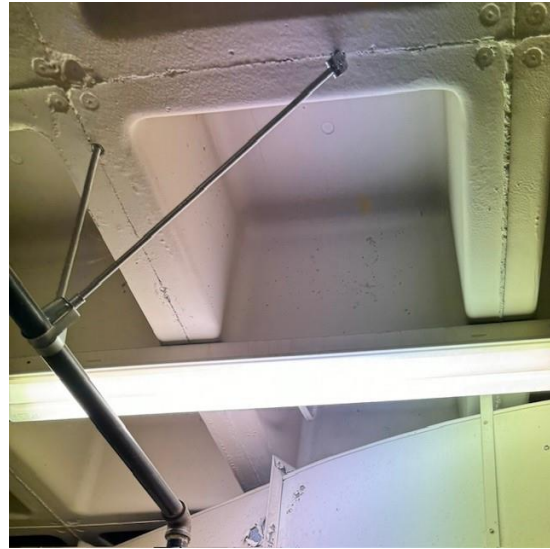
Photo #18 Asbestos-Containing Ceiling Coating (HA 43)
