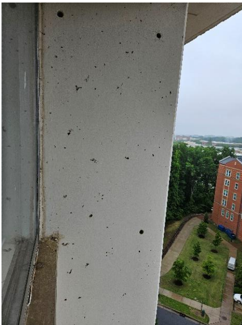
Photo #27 Asbestos-Containing Off-White Paint and Skim Coat (HA E1)
