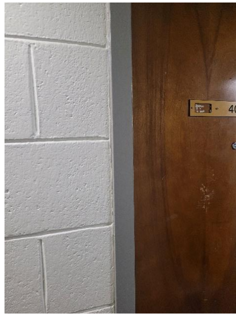
Photo #16 Asbestos-Containing Interior Door Caulk (Dorm Floors) (HA 39)
