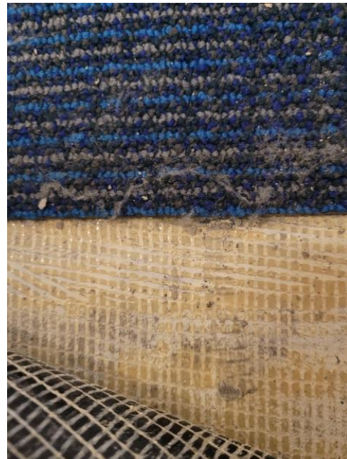
Photo #8 Asbestos-Containing 9"x9" Tan Floor Tile and Mastic (Under Carpet) (HA 26)
