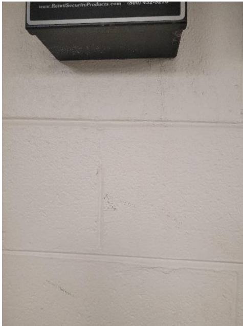
Photo #5 Asbestos-Containing CMU Block Surface Filler (Interior Stairwell) (HA 6)
