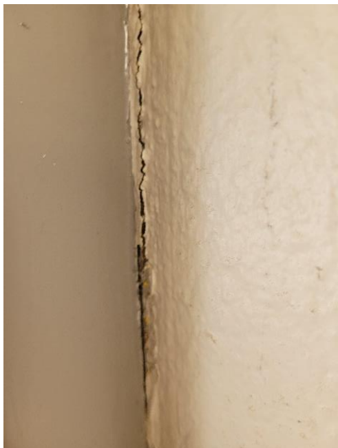
Photo #23 Asbestos-Containing Interior Window Caulk (Ground Floor) (HA 66)
