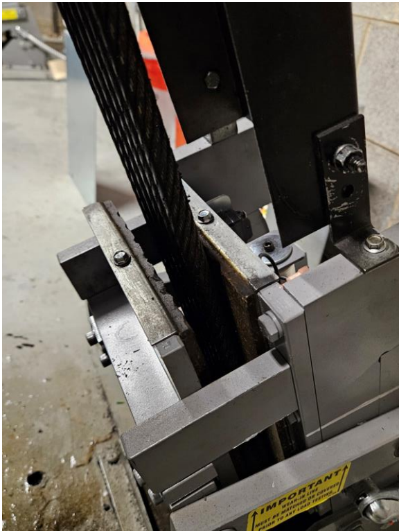
Photo #37 Assumed Asbestos-Containing Elevator Cable Brake Pad
