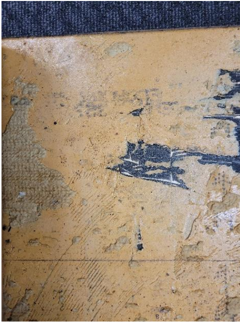
Photo #21 Asbestos-Containing 12"x12" White Floor Tile and Mastic (Under Carpet) (HA 64)
