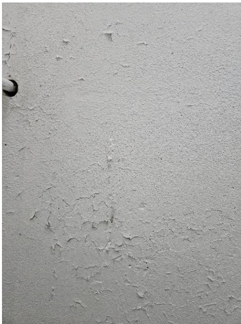
Photo #31 Asbestos-Containing White Ceiling Paint – Fire Escape Vestibules (HA E5)
